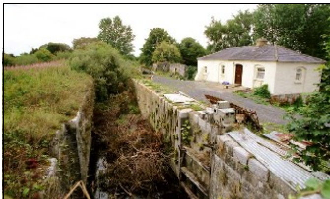
The abandoned first lock and still-inhabited lock-keeper's house on the Monasterevin-Portarlino road.
